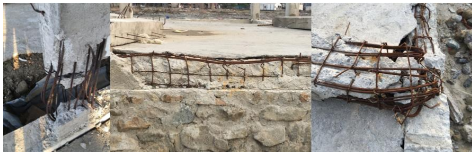
Figure 1. Improper Installation of Shear Reinforcement in Reinforced Concrete Beam-Column Members
